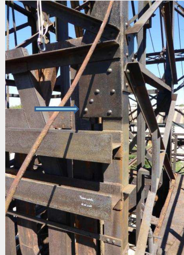
CORNERS OF THE FRAME MID OF THE SHAFT CHOSEN FOR LONG TERM EXPOSURE: TEST AREA CLEANED AND COATED WITH MICROCRYSTALLINE WAXES.
